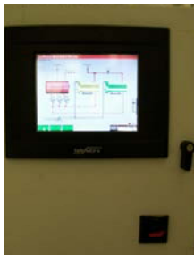
Energy management system
