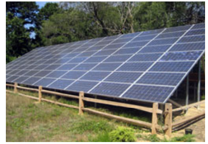
PV array, Wellfleet Wildlife Sanctuary, Massachusetts
