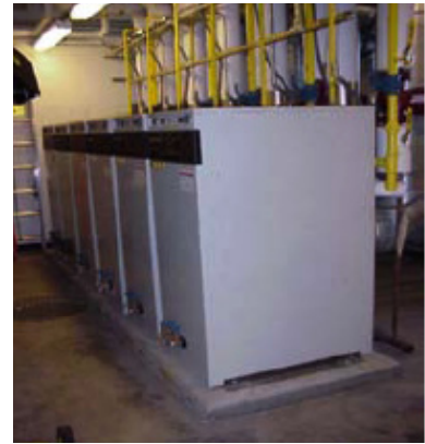
Modular boiler installation
