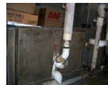
Flow balancing to a heating coil
