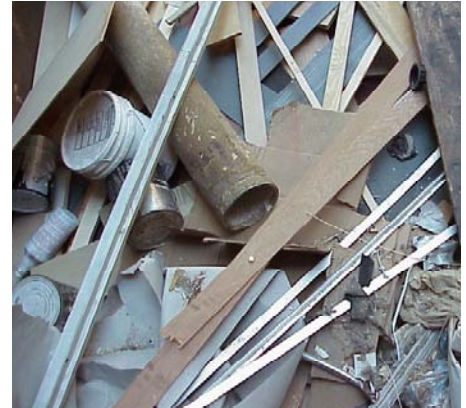
Comingled construction debris
